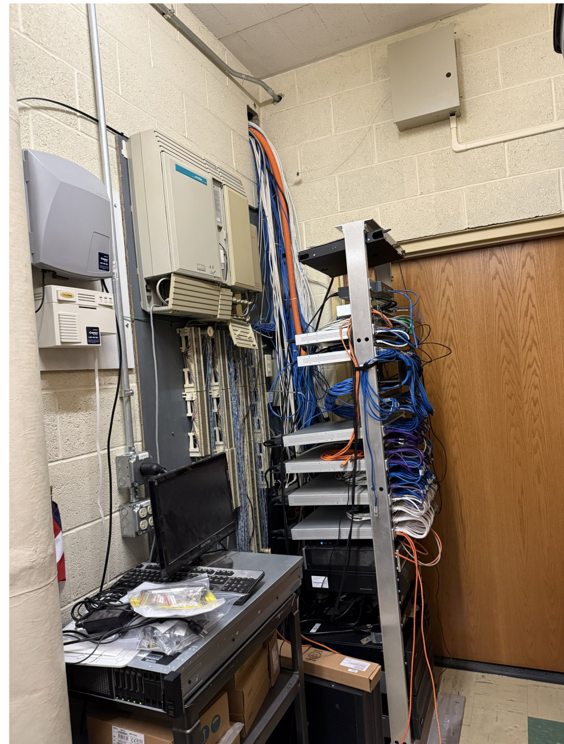
EXISTING DATA RACK TO BE REMOVED AFTER CUTOVER OF COMPLETE BUILDING TO NEW CABLING RACK SERVER IS TO INSTALLED IN NEW EQUIPMENT RACK
