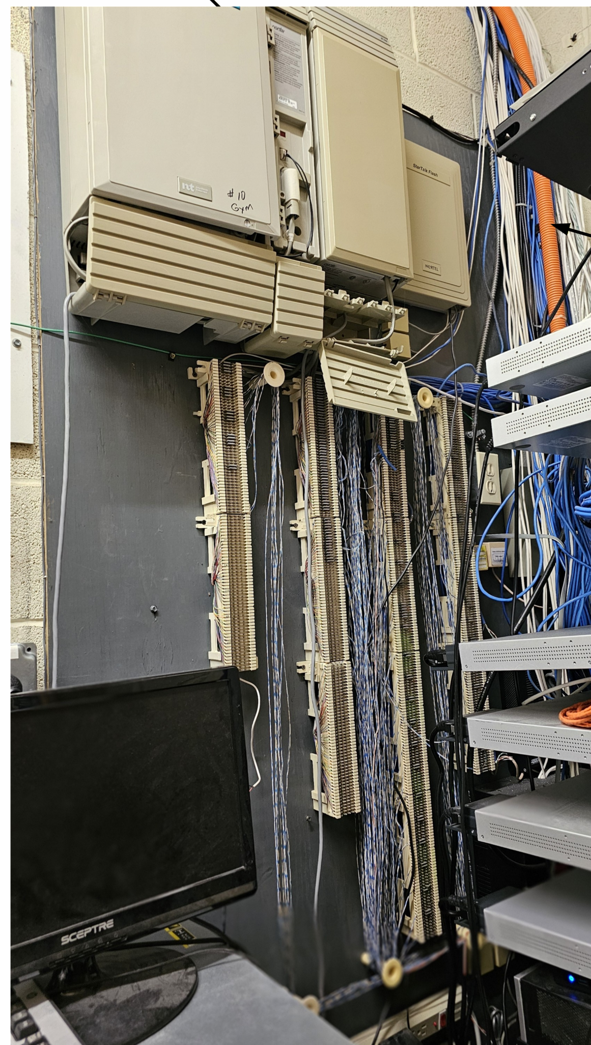
EXISTING LEGACY PHONE SYSTEM TO BE REMOVED INCLUDING ALL UNUSED TELEPHONE CABLING COORDINATE WITH OWNER TECHNOLOGY STAFF
